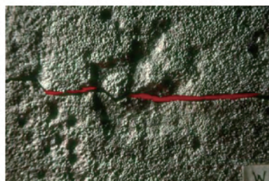
(a) 裂纹形貌
